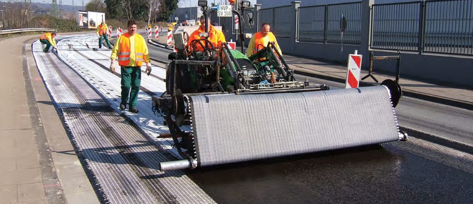
Mechanical installation of Tensar Glasstex is fast and efficient – an experienced crew can install up to 12,000m 2 per day, per tanker.
